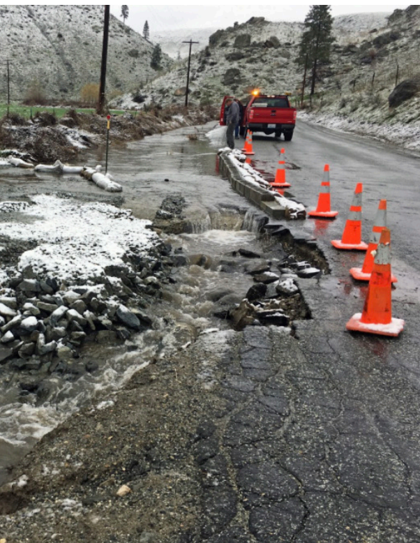
Flooding along Antoine Creek Road before culvert replacement. Photo Credit: Chelan County Public Works
