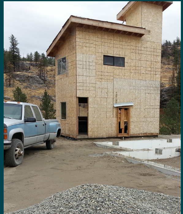
A rebuild underway in Okanogan County after the Carleton Complex Fire. Photo: Okanogan County Long Term Recovery Group (OCLTRG)
