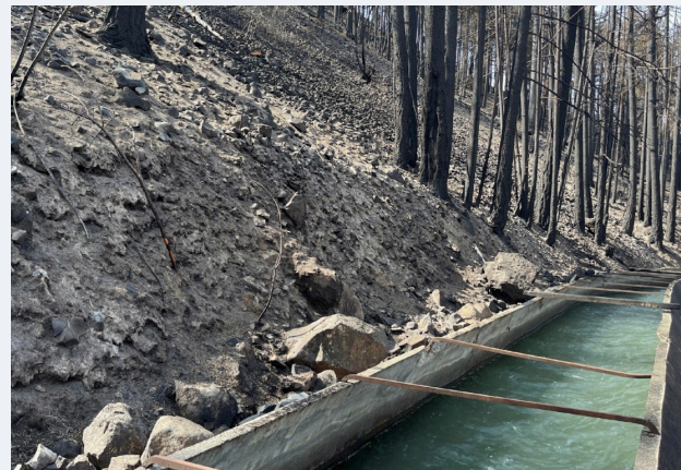
Slope stability is one of the primary recovery concerns as the already steep slopes have been weakened by debris flows. Photo Credit: Yakima Tieton Irrigation District
